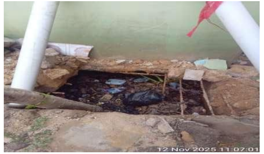
Picture showing a collapse septic tank of Household toilet in Awutu Beraku
